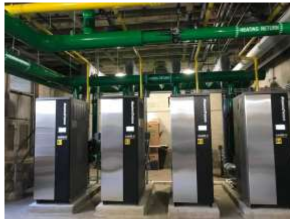
Possible New Boilers
